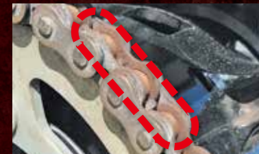
insufficient lubrication, roller wear
